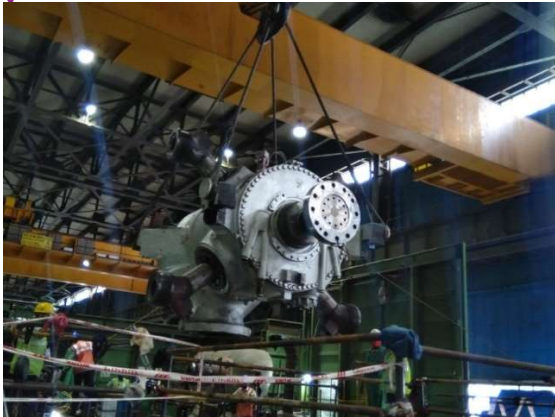
Refurbished HP turbine
