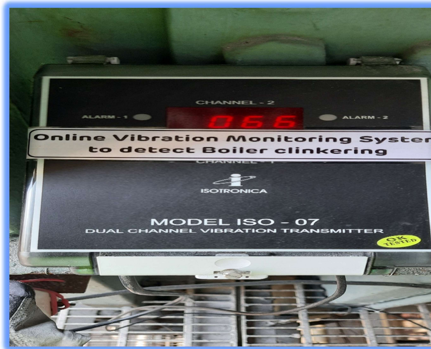
Online Vibration Monitoring of Boiler Clinkering
